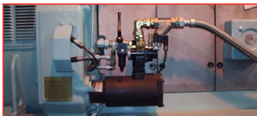
An ST400C03L94 mounted on a MAN B&W 16/24 marine generator set.
